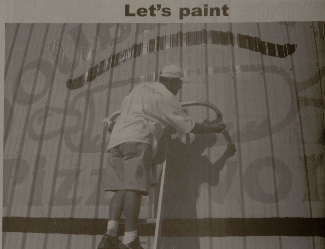
Cecil Garcia of Bryan paints a 15 feet by 10 feet logo mural onto the Double Dave's building located in Northgate on University Drive. Garcia and his crew will complete the mural with a second coat on Thursday.
