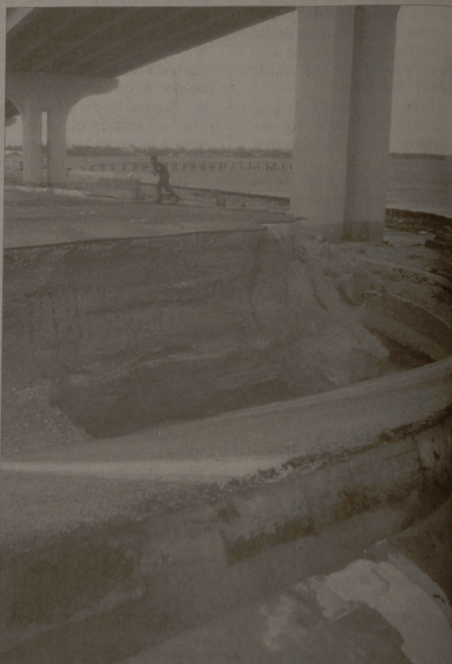
Department of Transportation workers survey the damage to the old Jensen Beach Causeway Sunday. Large portions of the road were washed away during Hurricane Jeanne.
