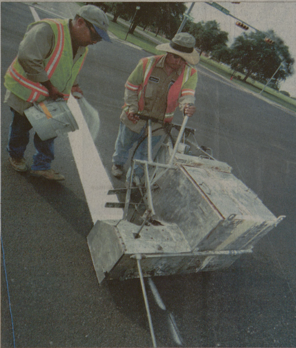
Alejandro Rocha coats newly-painted lines along George Bush Drive with highway safety spheres, or small spherical shards of glass as Jose Mendoza paints the lines. The glass acts as a reflective medium for driving at night.
