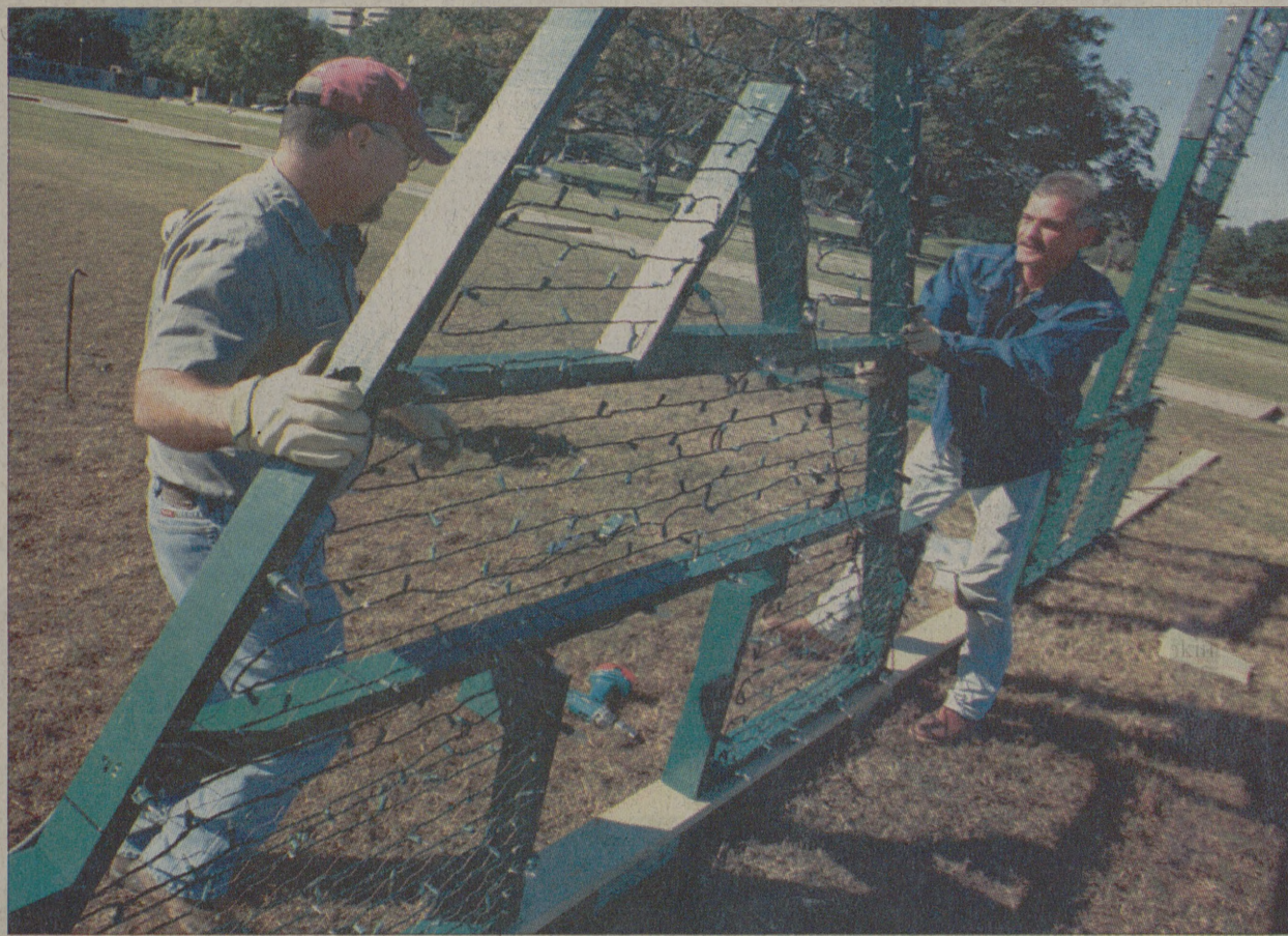
Charles Powley and John Coyle raise and secure winter holiday light fixtures in front of the Administration Building last week. The fixtures were funded by the A&M Physical Plant.
