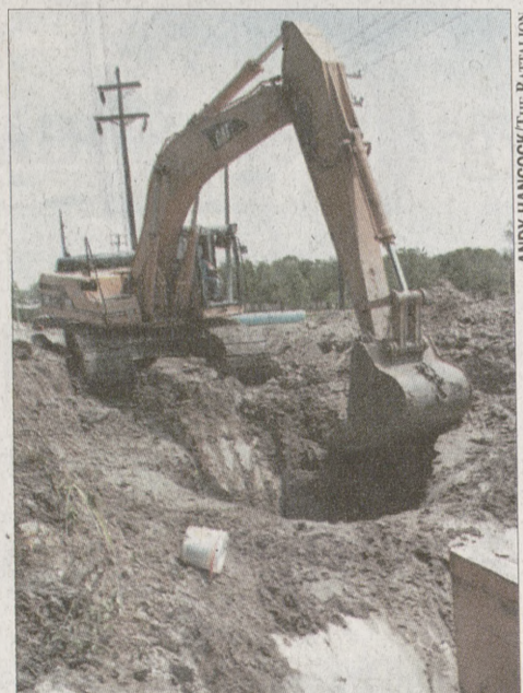
The Domestic Water System Improvement Project is in the process of upgrading the waterlines that run through campus.
