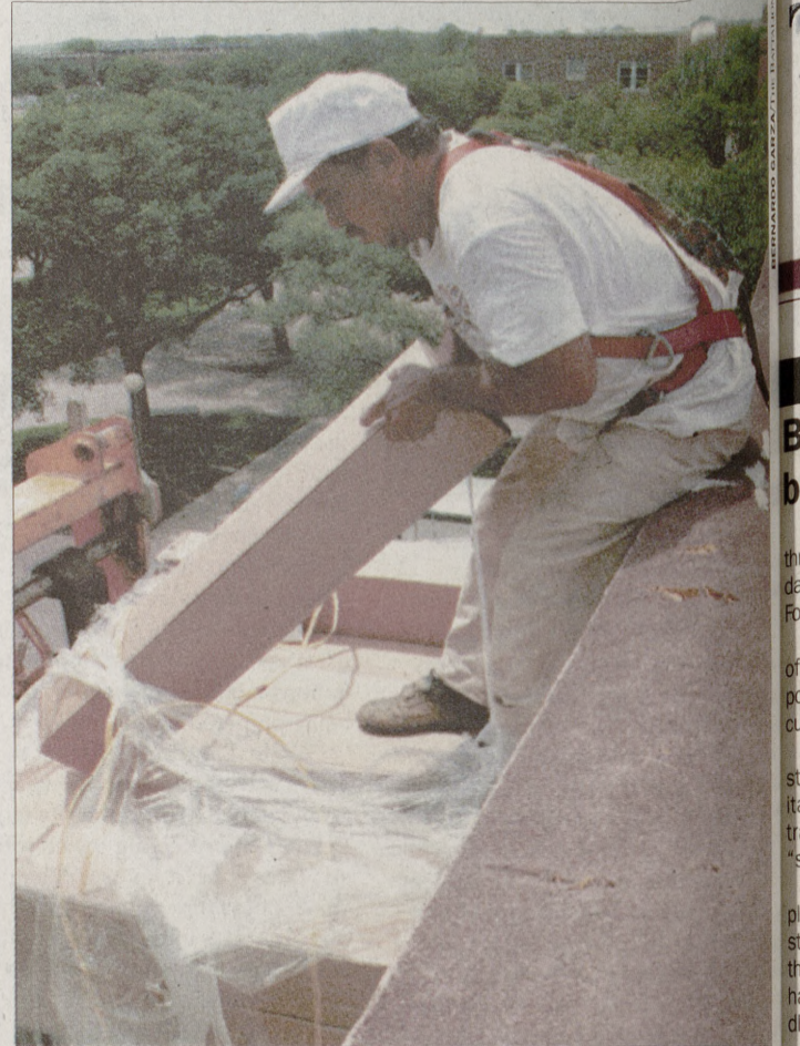
Construction worker Nero Rios unloads material to repair the roof of the MSC.
