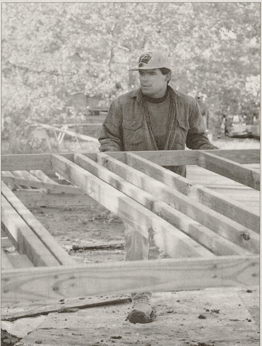
Anthony Jaime, a new Habitat for Humanity home recipient works to raise the walls of his home on June Street in Bryan Saturday morning. The house is the fifteenth home built by Habitat on June Street and the walls were raised as part of a ceremony.
