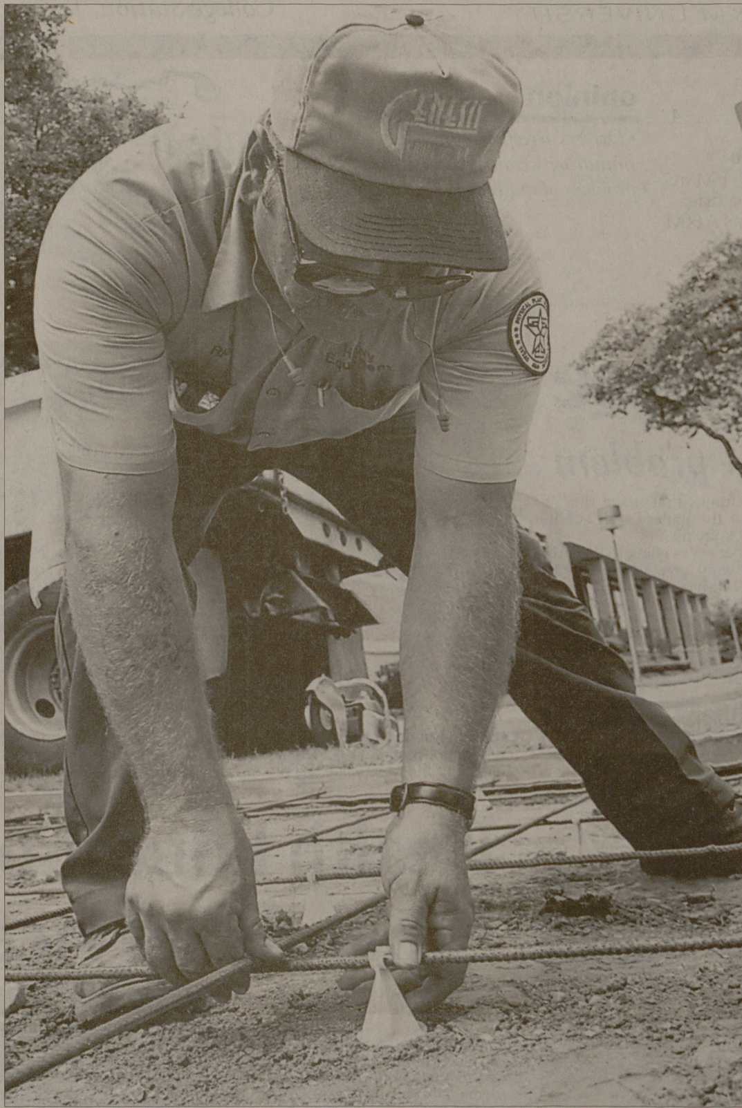
Richard Levan of Heavy Equipment places spacers under the reinforcement rebar before laying concrete for the sidewalk at the corner of Throckmorton Road and Joe Routh Boulevard Wednesday. The sidewalk needed repair after it was washed out.
