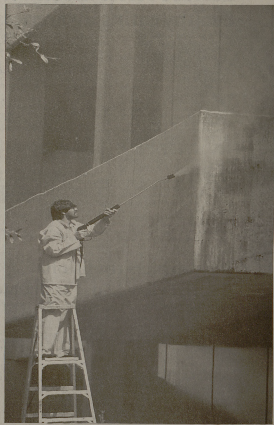
JP BEATO/THE BATTALION Arthur Kaml, a University employee, uses a pressure washer to clean the rear of Rudder Tower. The water has a force of 3,500 pounds per square inch.
