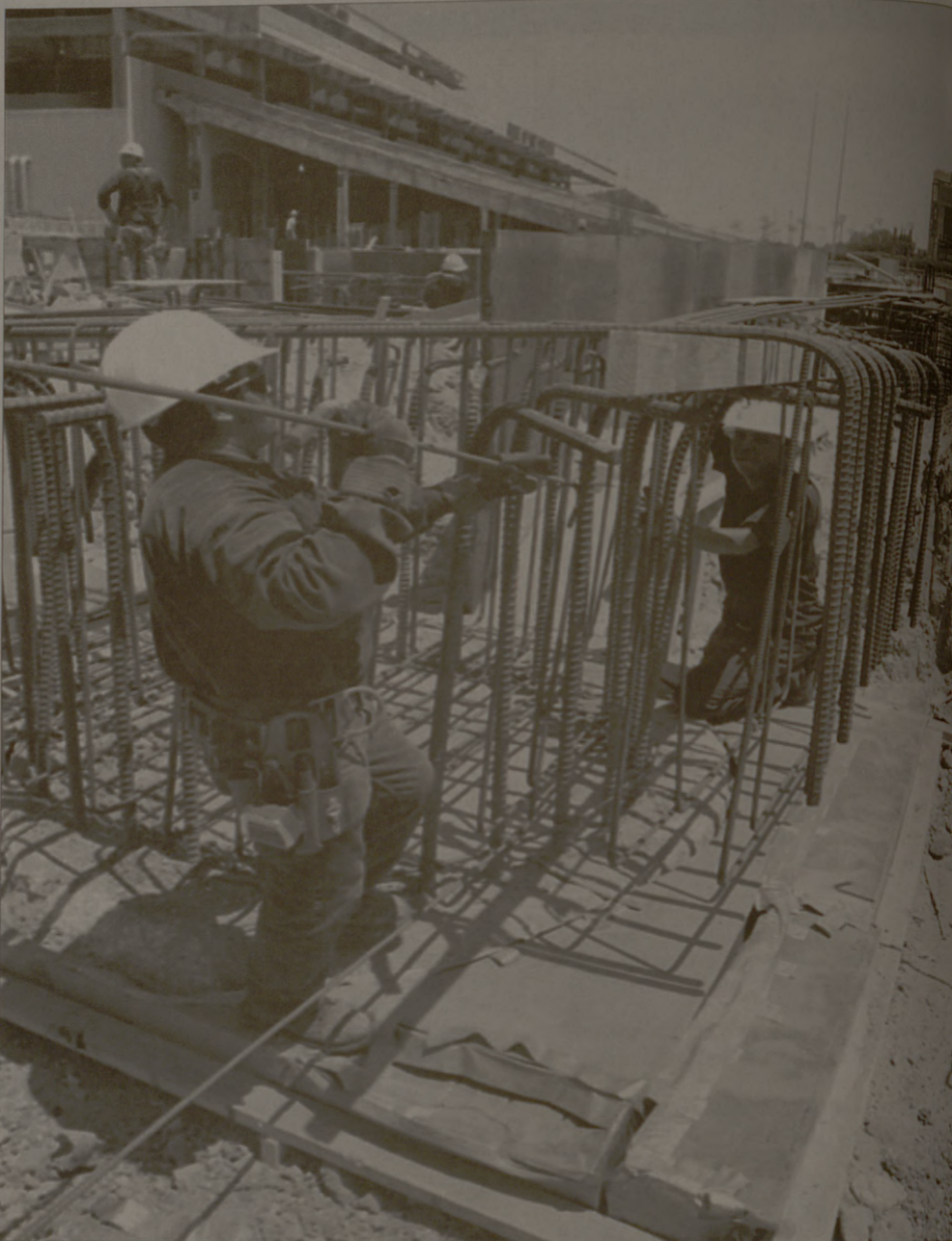
Jose Sotolo (left) and Ruben Bartos (right) assemble rebar forms for columns at the Kyle Field construction site Monday afternoon.
