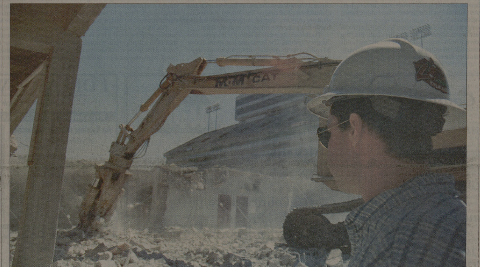
Randall Jay, an assistant superintendent for Bartlett and Cocke Construction, oversees the demolition of part of the horseshoe of Kyle Field Saturday afternoon.
