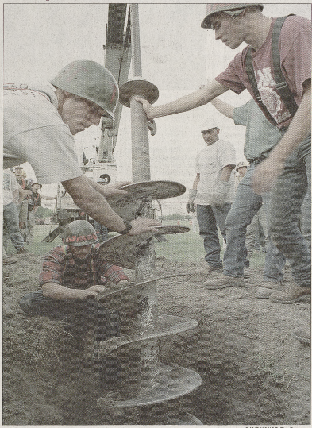
Junior redpots T.J. Saari, an agriculture business major, Gabe Perez, a construction science major, and Nathan Buschow, a general studies major, set the drill to dig a hole Wednesday for one of Bonfire's four perimeter poles.
