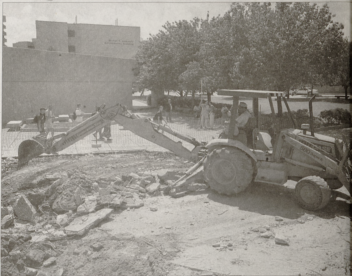
Workers remove soil in front of Blocker after compacting caused sidewalks to fracture.
