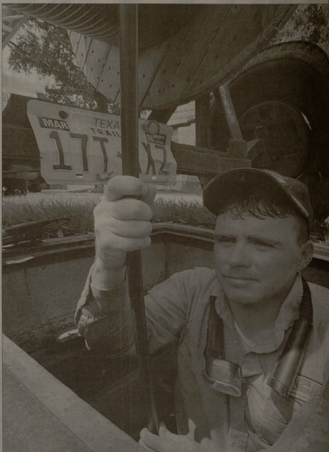
Cable Guy Jerry Webb, a TCA cable construction worker, hooks up fiber optic cables in front of Corps dorms Tuesday. The cables will improve modem operations on campus.
