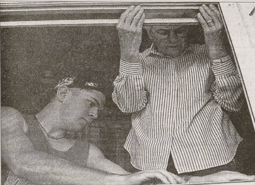
From top: (top) Kyle King, a senior construction science major, puts the last nail in a porch he built with other National Association of Homebuilders members; (middle) David Gunn, a senior construction science major, puts a coat of paint on the porch; and (above) Jeremy Marshall, a freshman business administration major, helps Mrs. Mainer install a window screen after workers cleaned her windows.
