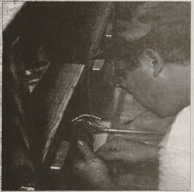
Nick Rodnicki/THE BATTALION Robert Milford, a worker for Britt Rice Electric works on the Underground Monday.
