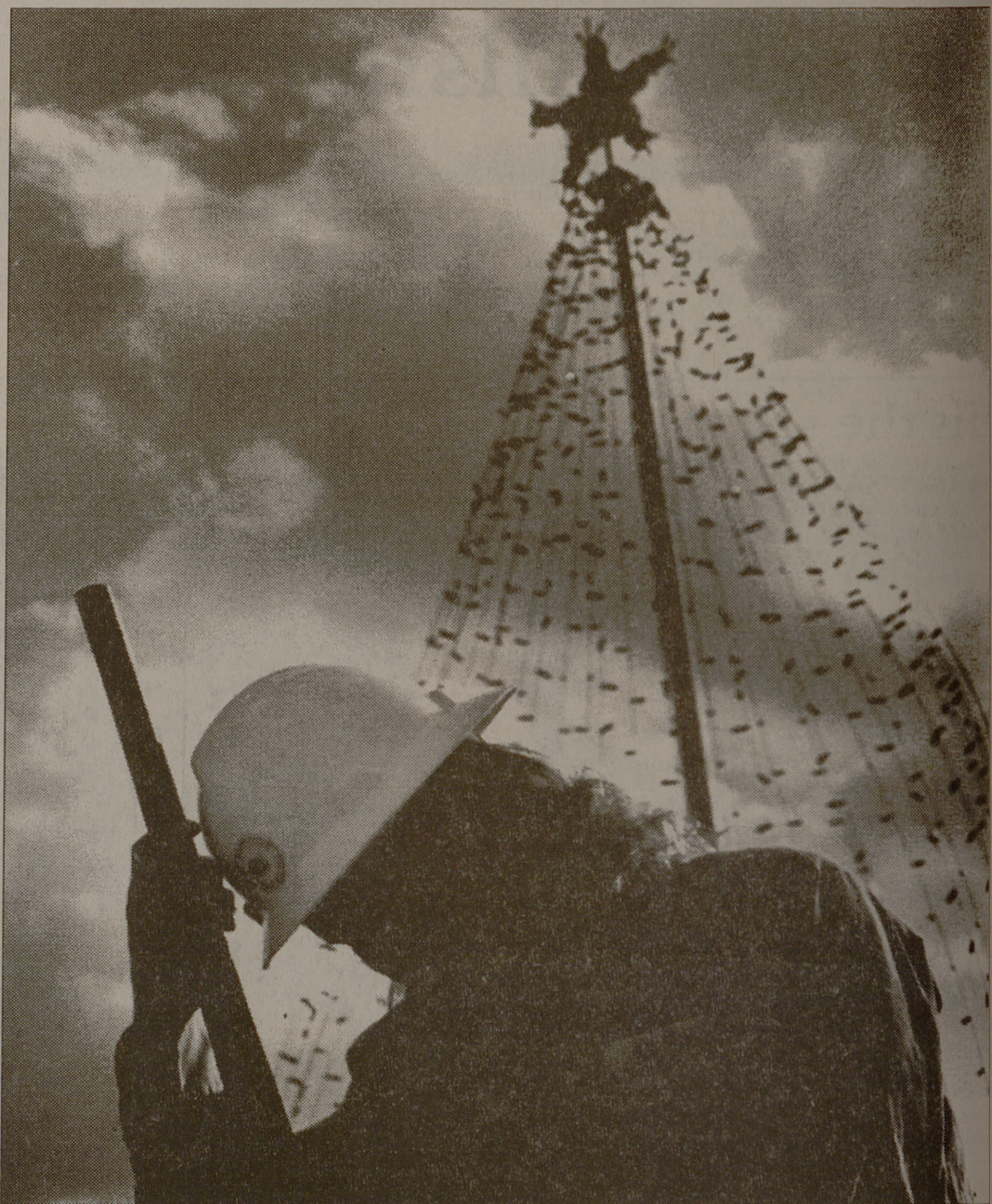
Chris Colloway, with the City of College Station electrical department, works on the community Christmas tree Tuesday at the intersection of Texas Avenue and University Drive.
