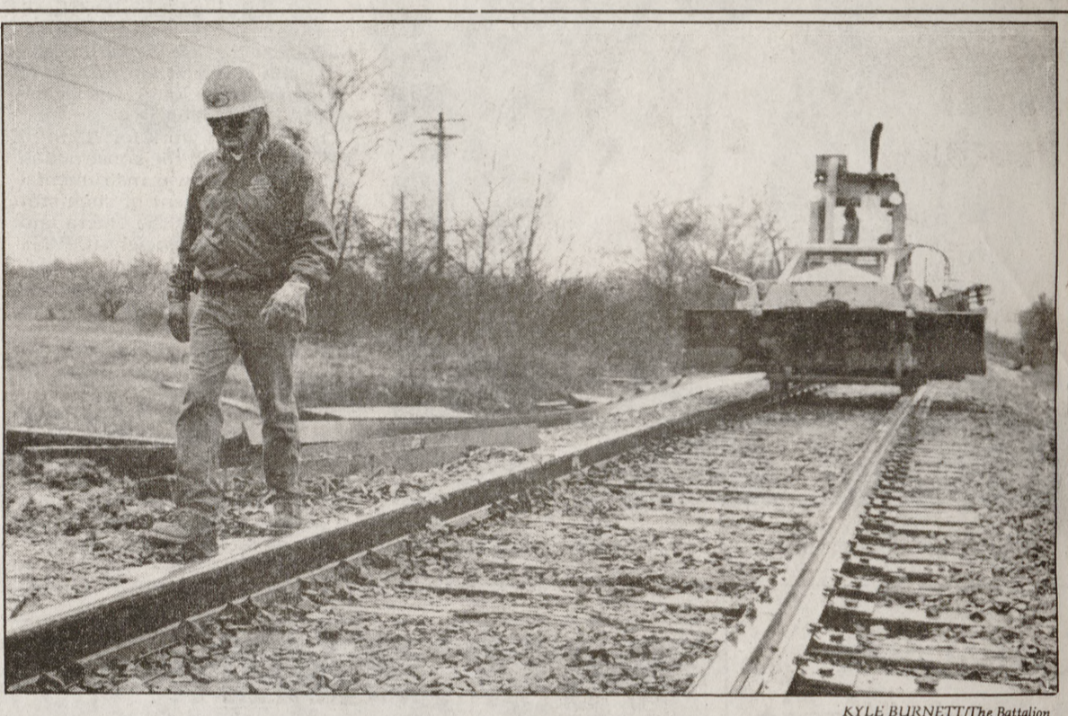
An unidentified construction worker continues work on the railroad tracks near FM 2818 and Wellborn road. Recent rains have delayed completion of the project thus restricting traffic.
