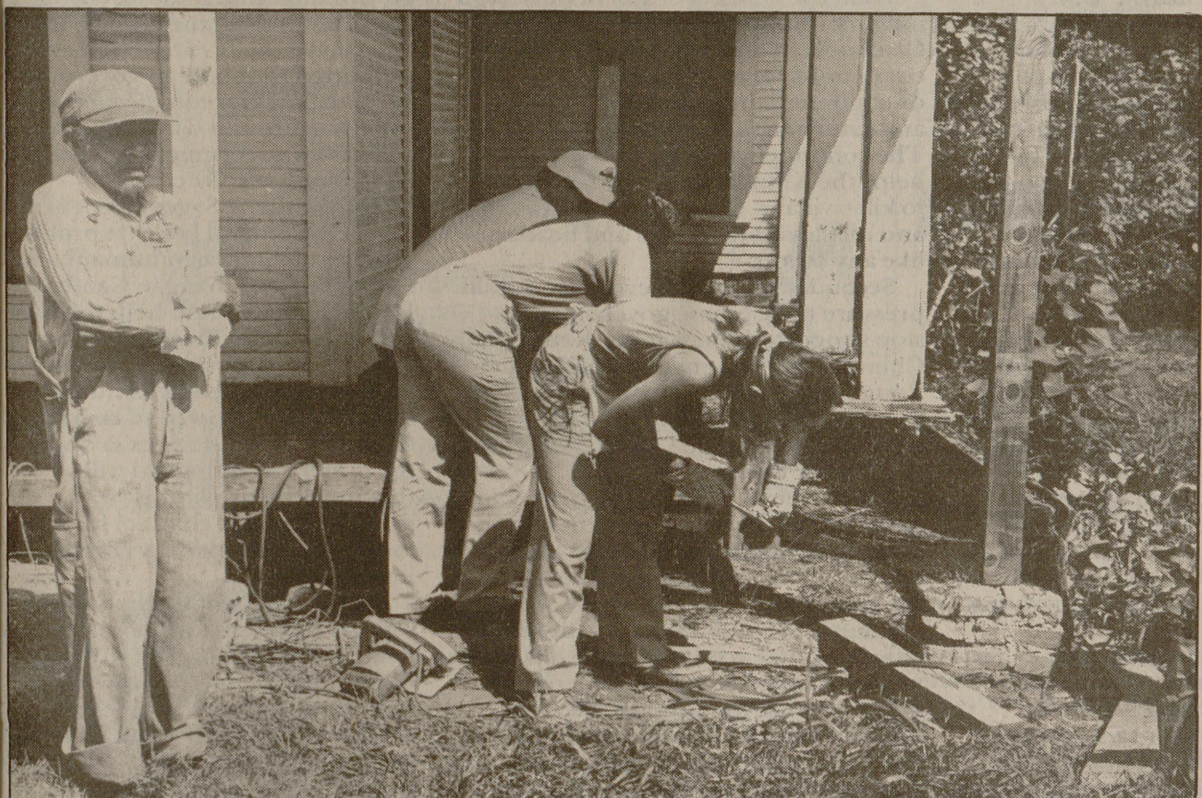
A group of Federal Prison Camp inmates volunteers its time and labor to repair the home of 88-year-old Dyas Hicks (left) as part of the Prison Fellowship ministry, aimed at providing services to the community. Work on the home began on July 26 and is expected to be completed July 28.
