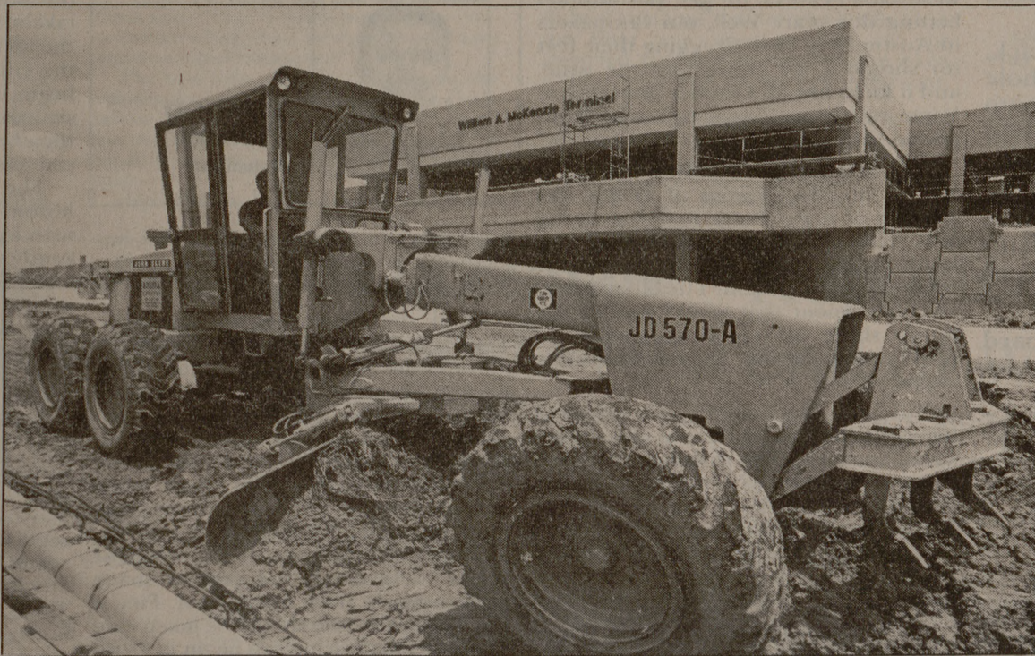
Construction continues on the William A. McKenzie Terminal at Easterwood Airport. The
