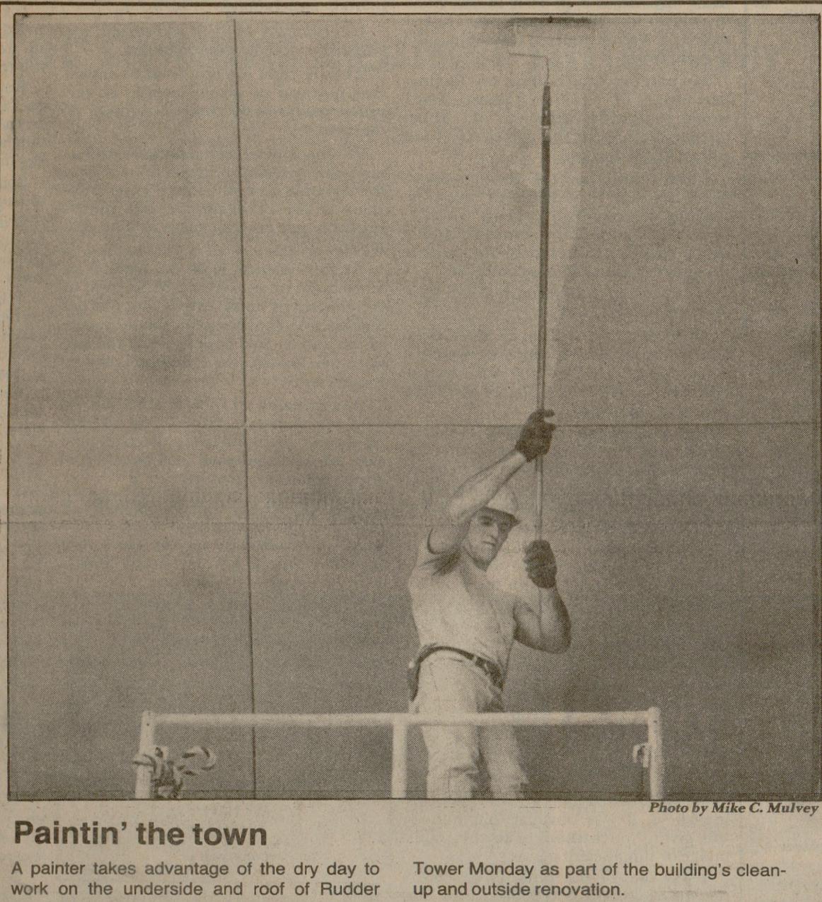
Paintin' the town A painter takes advantage of the dry day to work on the underside and roof of Rudder Tower Monday as part of the building's clean-up and outside renovation.
