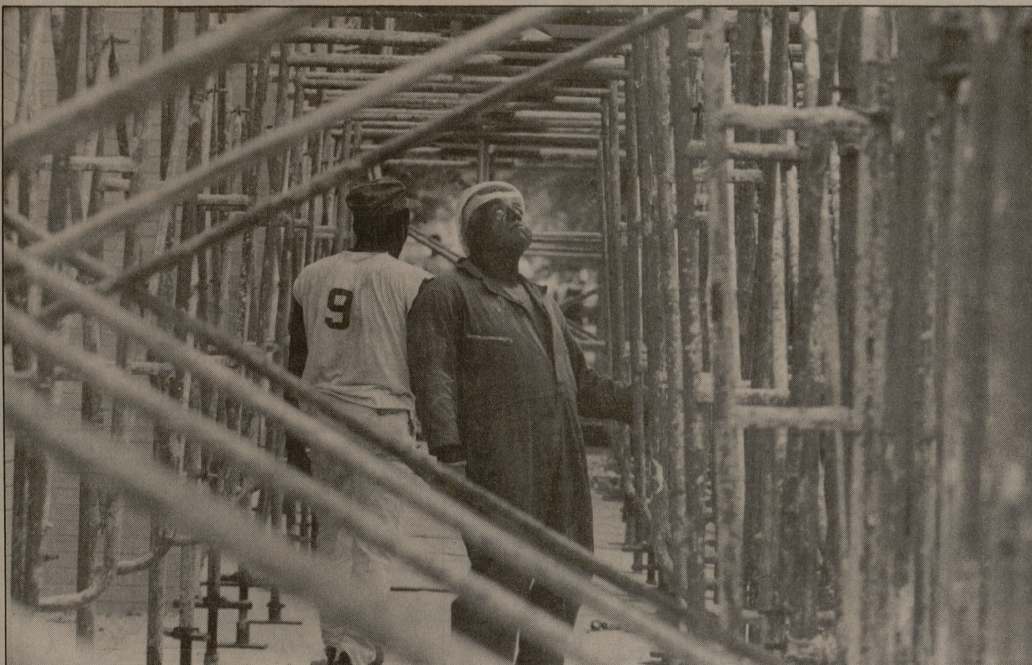
Construction workers inspect scaffolding Thursday after trimming trees to clear the way for repair on the north side of Sterling C.
