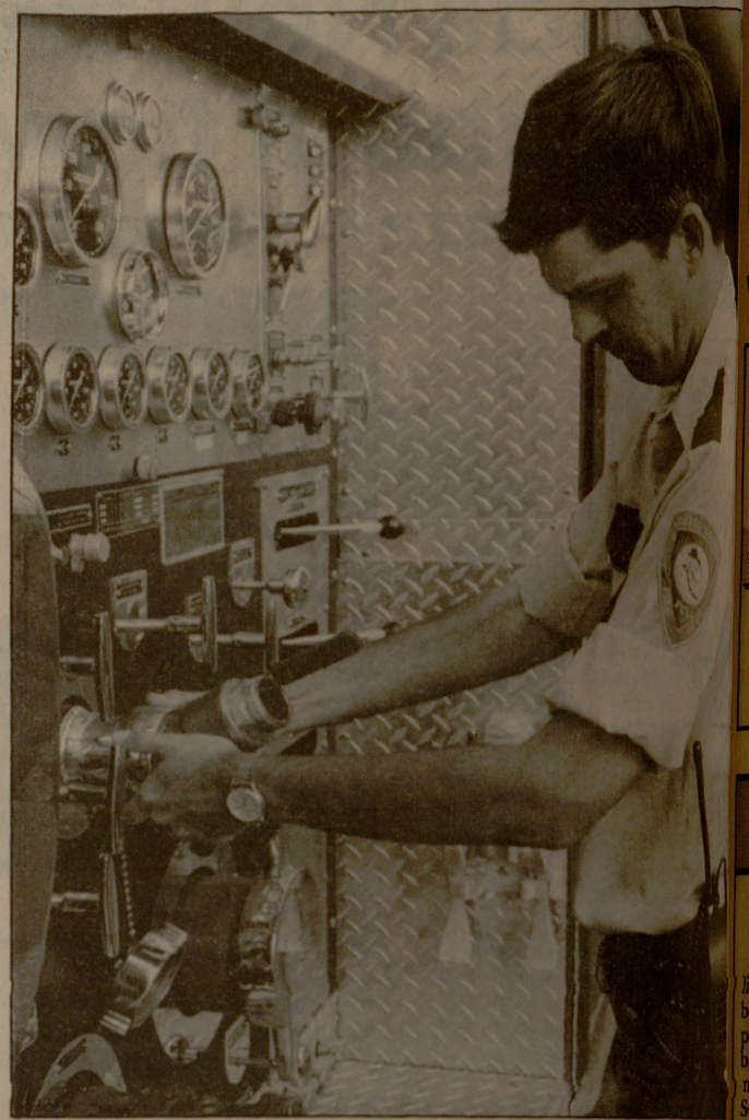
Fire Chief Mark Lenz checks the pumps on one of the fire trucks.
