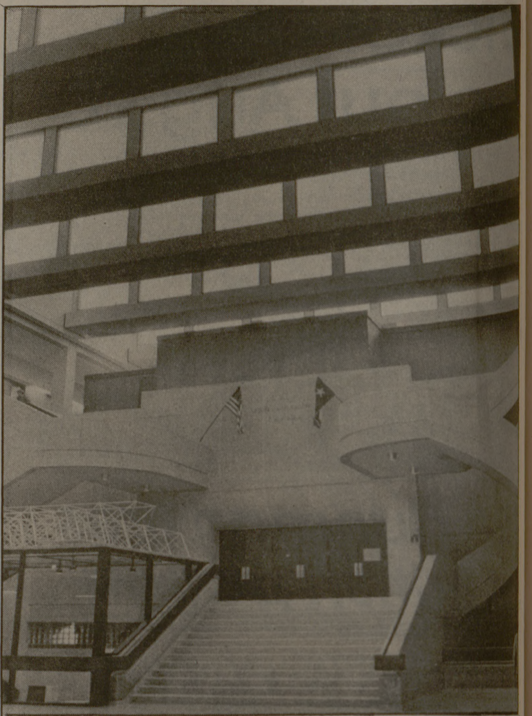
Skylights such as these in Zachry Engineering Center may help increase energy efficiency.
