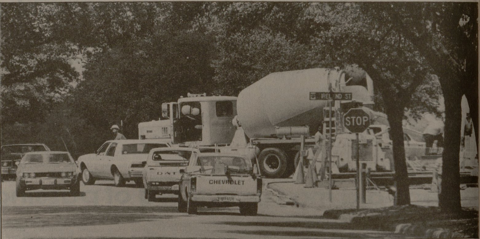
Campus traffic was temporarily hampered Wednesday afternoon near the intersection of Ross and Ireland Streets by a cement truck which blocked half the street while making a delivery. The cement was used in the construction of a new manhole which will better facilitate the repair of underground telephone wires.
