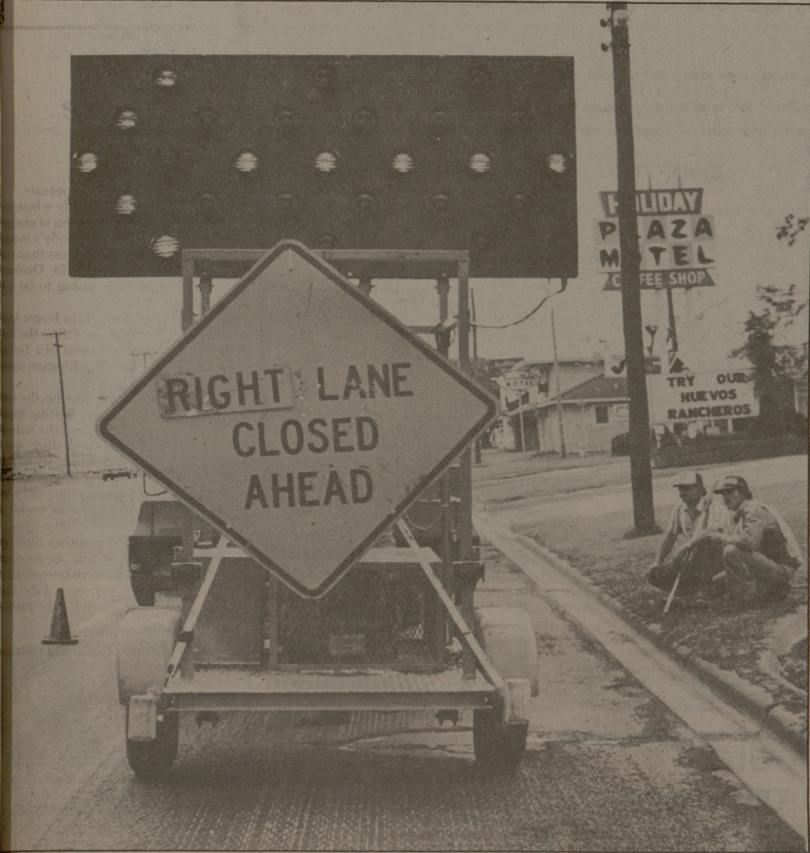
Lanes of Texas Avenue have been closed to traffic to allow workers to clean them. The work is being done preparatory to resurfacing 5 miles of the street. Battalion photo by Sam Stroder
