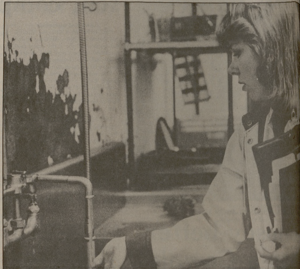
Ruth Maddox checks the hot and cold running water in "Restaurant B." Despite what were apparently much more severe violations than "Restaurant A," there was only a difference of one point of 100 possible between the two.
