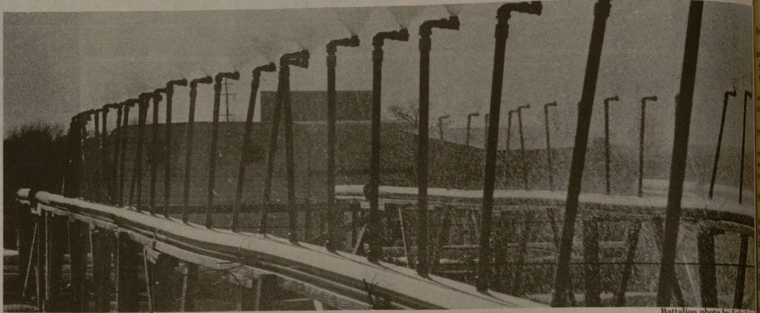
A sprinkler system sprays water so air can cool it. It will be pumped underground and used for cooling this summer.
