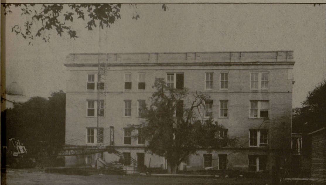
Cranes and fences are evidence of renovation now taking place at Legett Hall. The hall may become a women's dorm.
