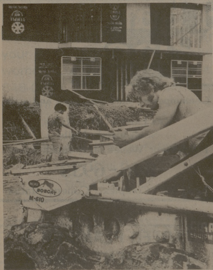
Battalion photo by Ed Cunniss Winston Simms, foreground, works to complete the Timber Ridge apartment complex, one of three which wasn't finished on schedule.
