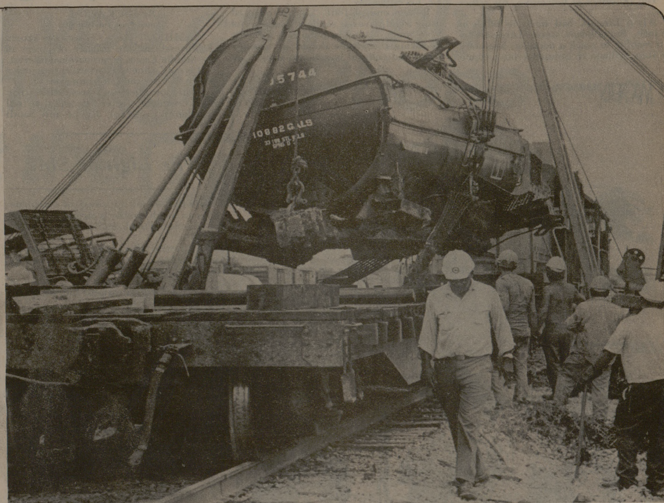
Southern Pacific Railroad workmen load a mangled railroad tank car onto a flat-bed car, to move it from the site north of the Texas A&M campus where nine Southern Pacific cars derailed Monday. Southern Pacific officials
