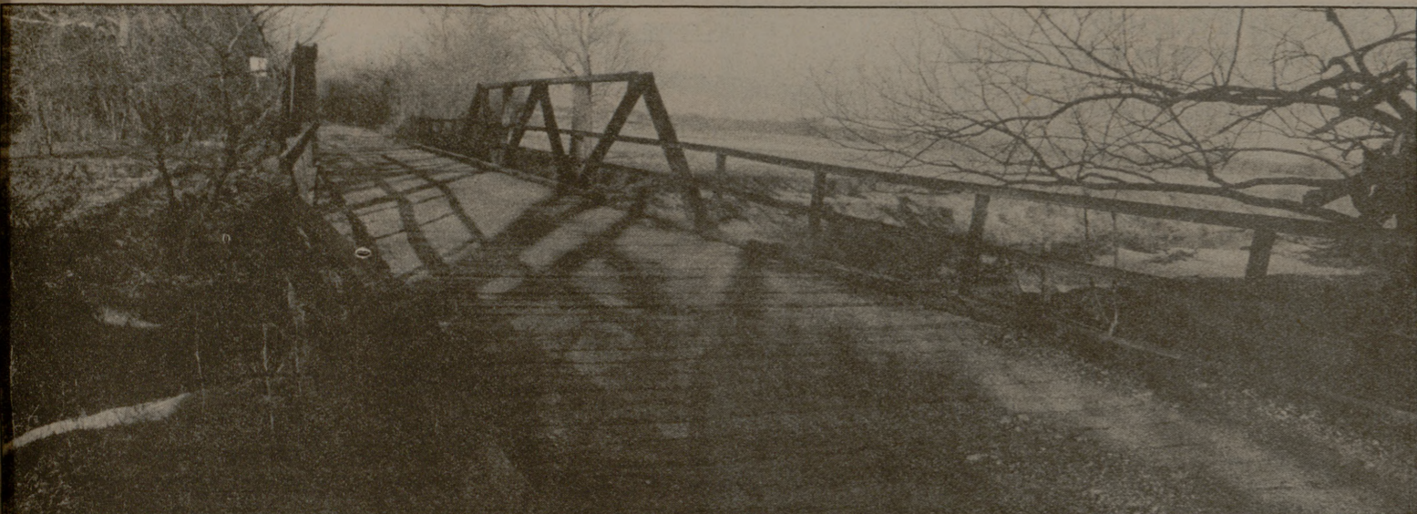
Driving along the country roads of Brazos County, one might run across a picturesque one-lane bridge. Many of the county-maintained bridges are made of wood with steel reinforcement like this one on Bird Pond Road. Some of the
