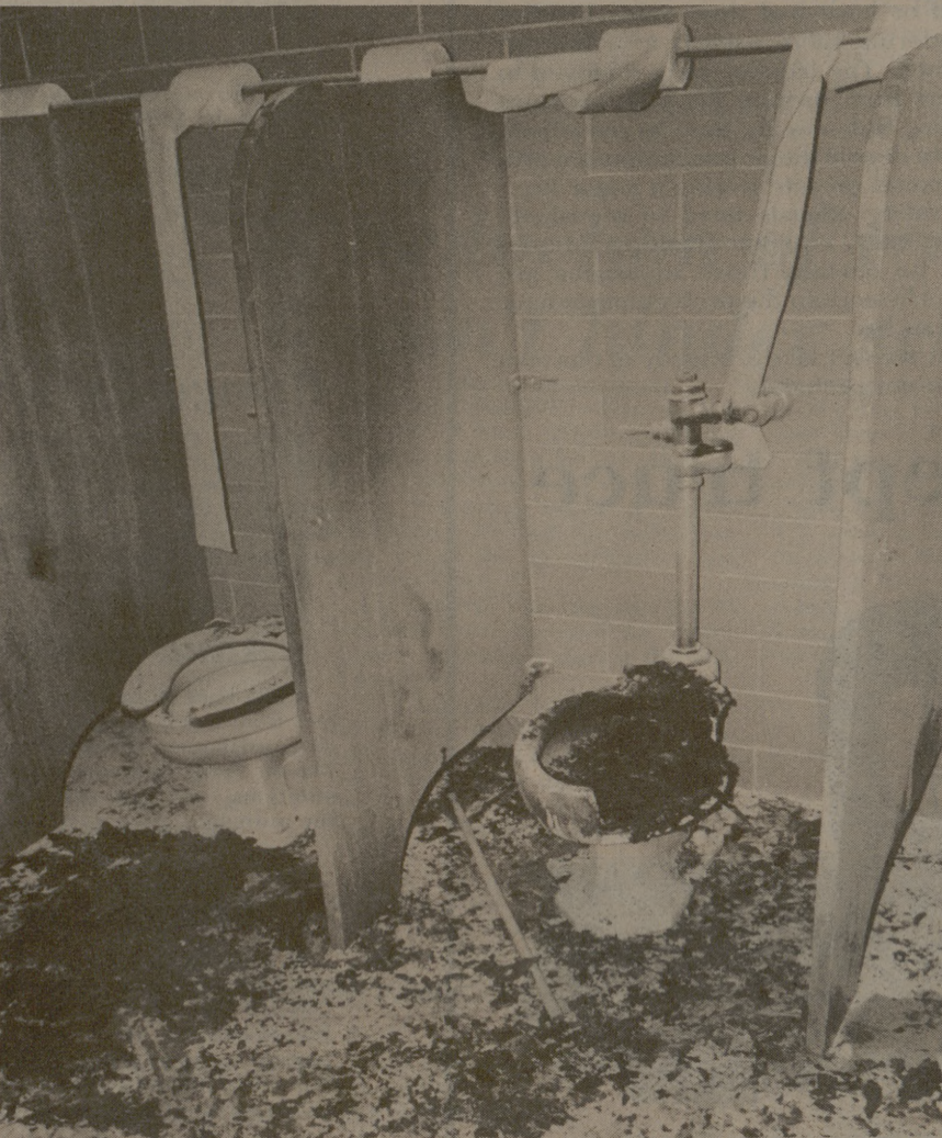
A fire yesterday morning about 4 a.m. destroyed a toilet seat in Dorm 8. The toilet area on the fourth floor was filled with melted trash containers and burnt papers.
