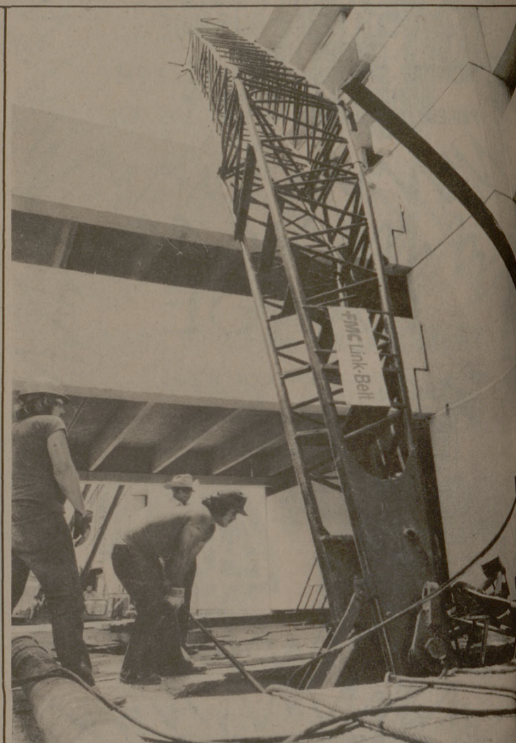
unless the ground shifts under the crane. When it did last spring at the Soil and Crop Sciences building site, the boom snapped off and made a hole in the building's floor.
