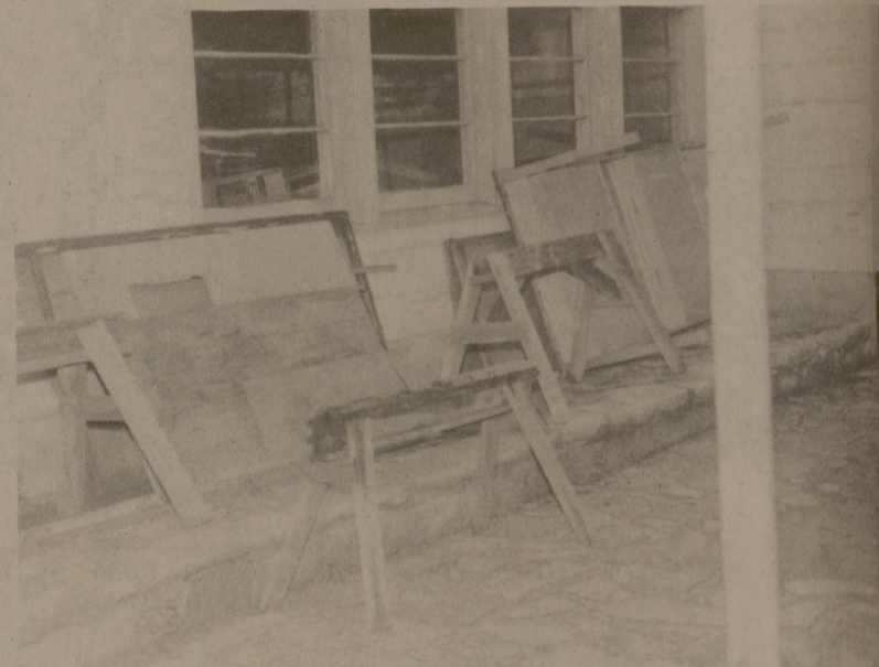
This is a view of one of the older six classroom buildings now being used for storage and maintenance work. The present Bond issue proposes to demolish the building; I say it can be restored and used, but the maintenance personnel certainly need a more adequate place for storage and working.
