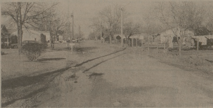
Construction of curbs and gutters on Sterling Street in southeast College Station is scheduled to begin next week under the Community Development Plan. Other city streets will also be renovated through the federal program.
