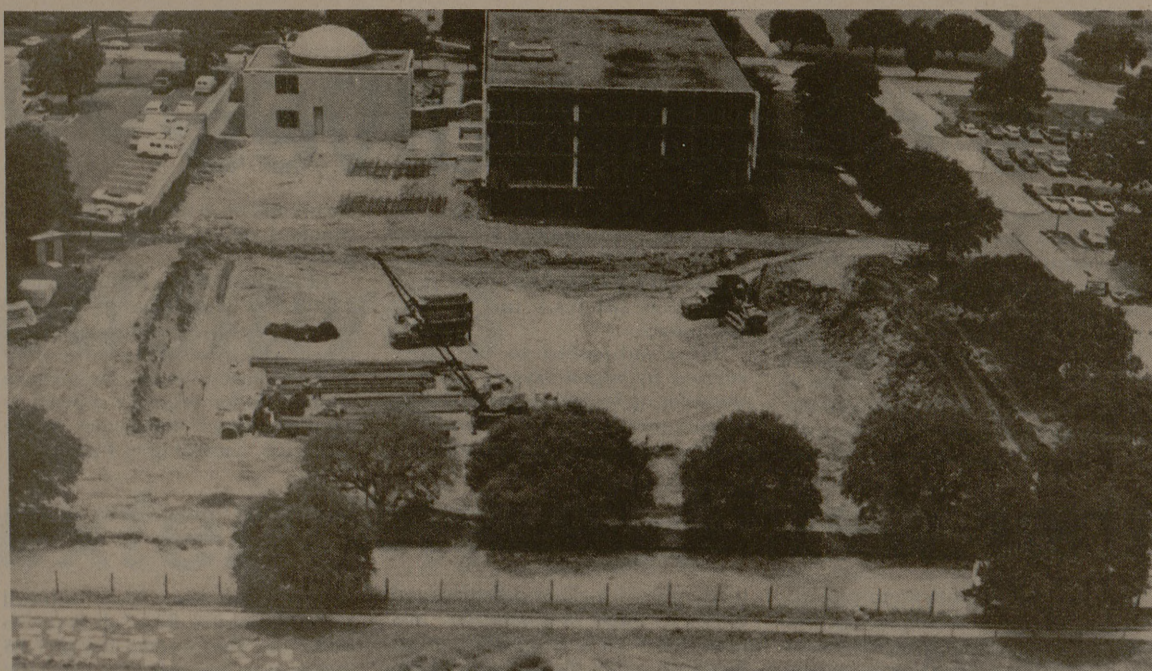
Taken from the top of the Oceanography-Meteorology building, the above picture shows the excavation site for the foundation of the new Architecture building. The building will be adjacent to the old Architecture building located top center in the photo.
