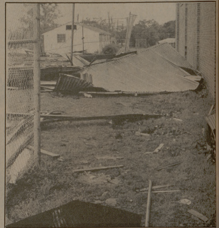
The roof of the Calvert High School gym. A National Guardsman remarked that it was "sheared off like a putty knife." It was the last place hit in the town.
