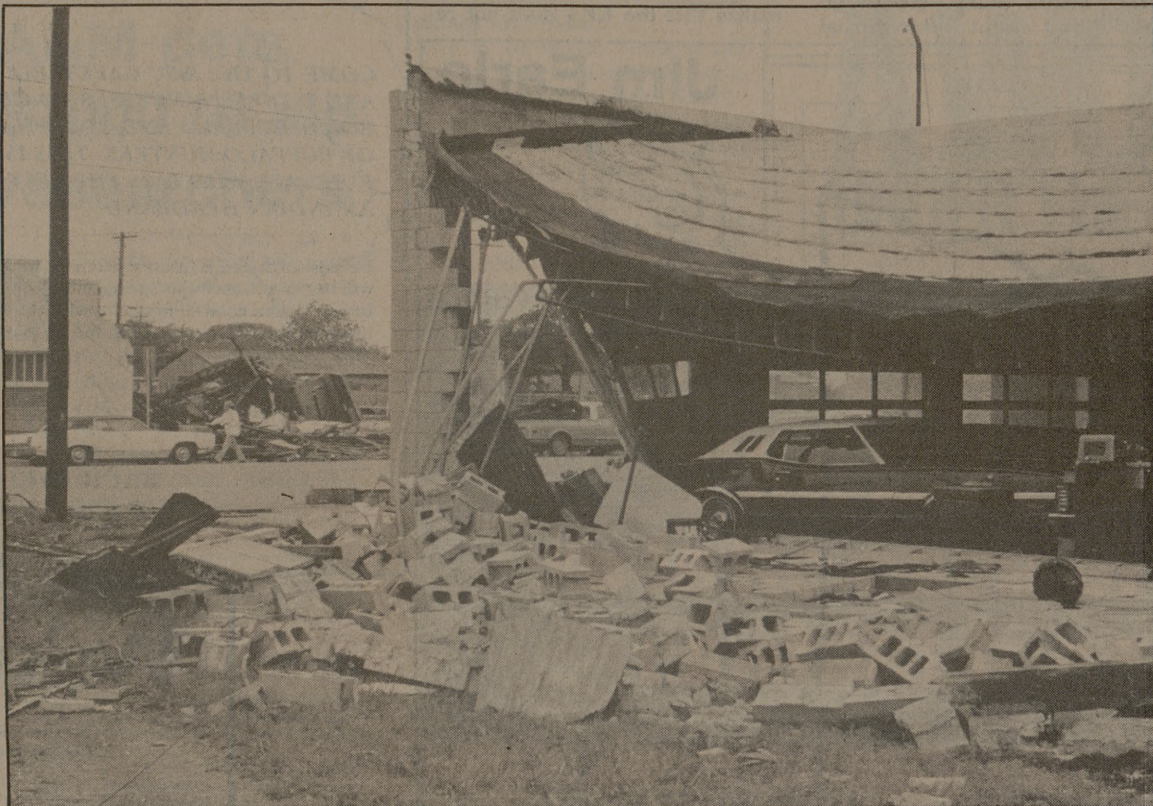
Fontana Ford Co. in Calvert suffered extensive damage when the twister dipped out of the southeast damaging several buildings in the downtown area. Photo by Alan Killingsworth
