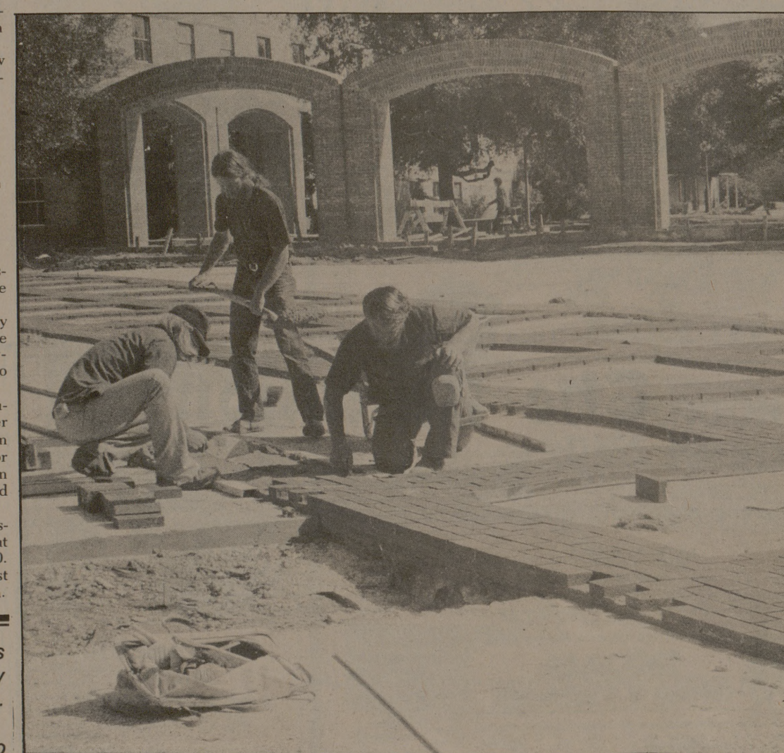
Tiles fall in place Renovation of Corps dorm area includes a sidewalk made of tiles. Workers are about to complete this part of the construction, and will go with arches and cement walks.
