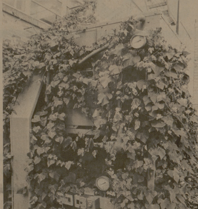
This condenser, with gauges and buttons peeking out, makes a hefty latticework for the vines that have heavily entangled it on campus.
