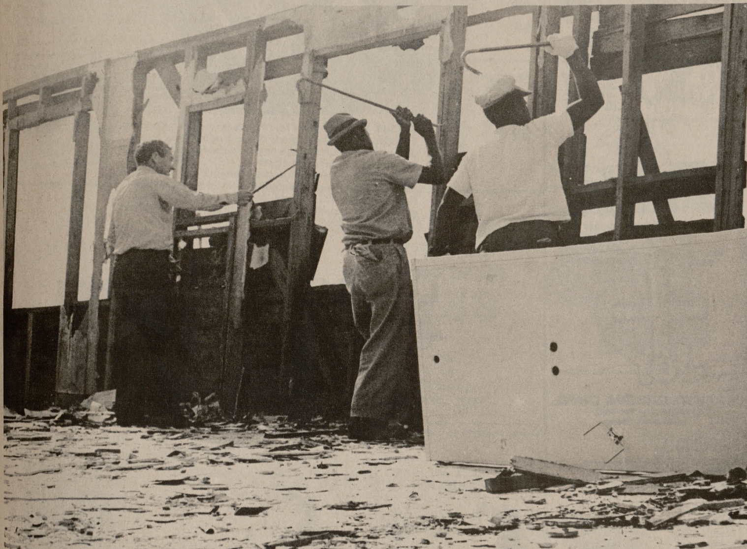
HENSEL PARK APARTMENTS are being torn down as part of a renovation program passed at the last Board of Directors meeting. (Photo by Nancy Swan)
