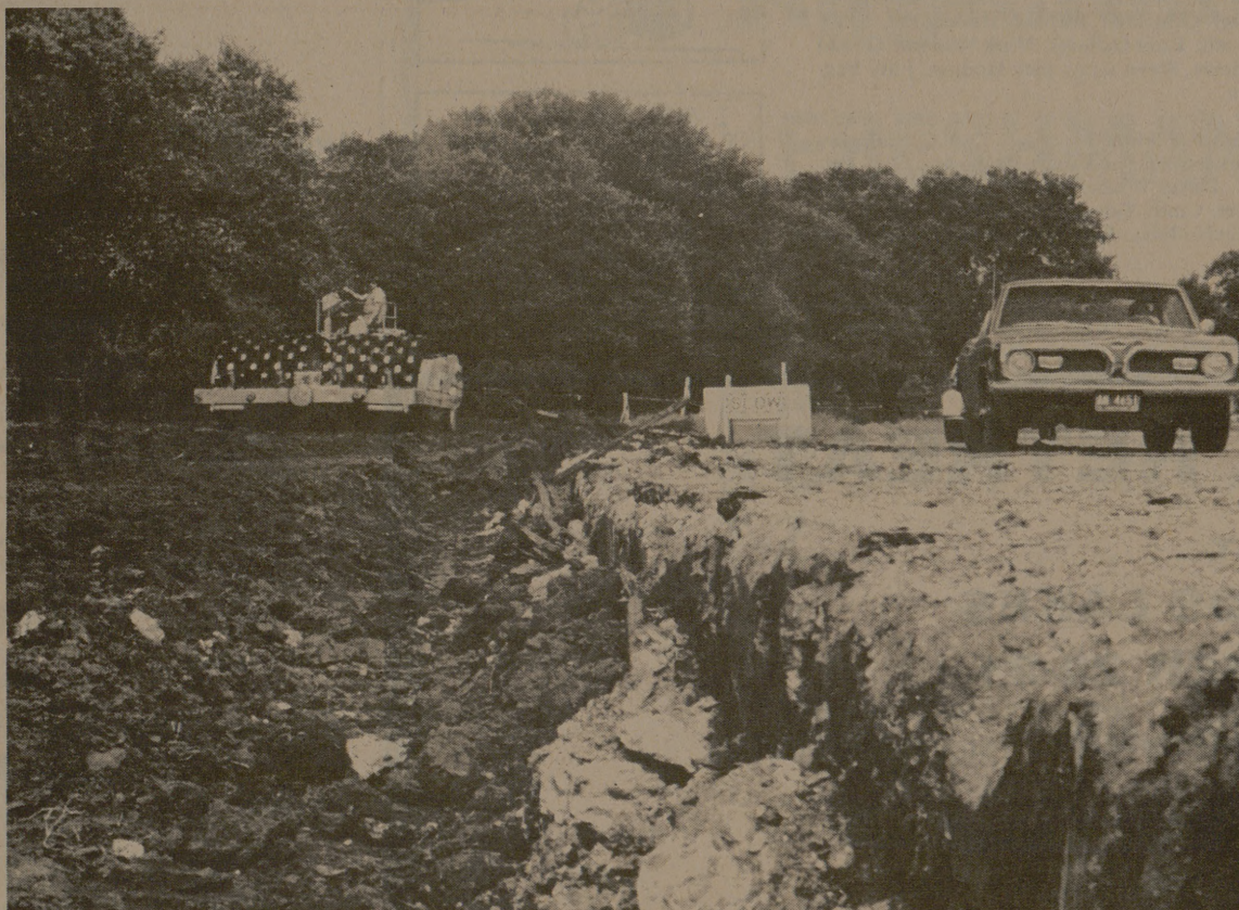
CONSTRUCTION OF A FOUR-LANE street in front of the Systems Building is back in progress after the rains. (Photo by Douglas Winship)
