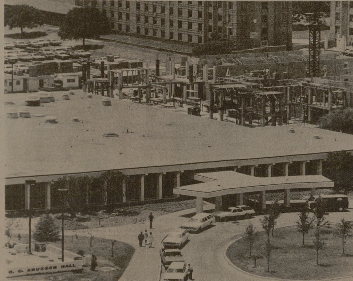
TWO NEW WINGS to the Krueger-Dunn complex now under construction will house an additional 1158 students in the fall of '75 at a cost of $10 million.
