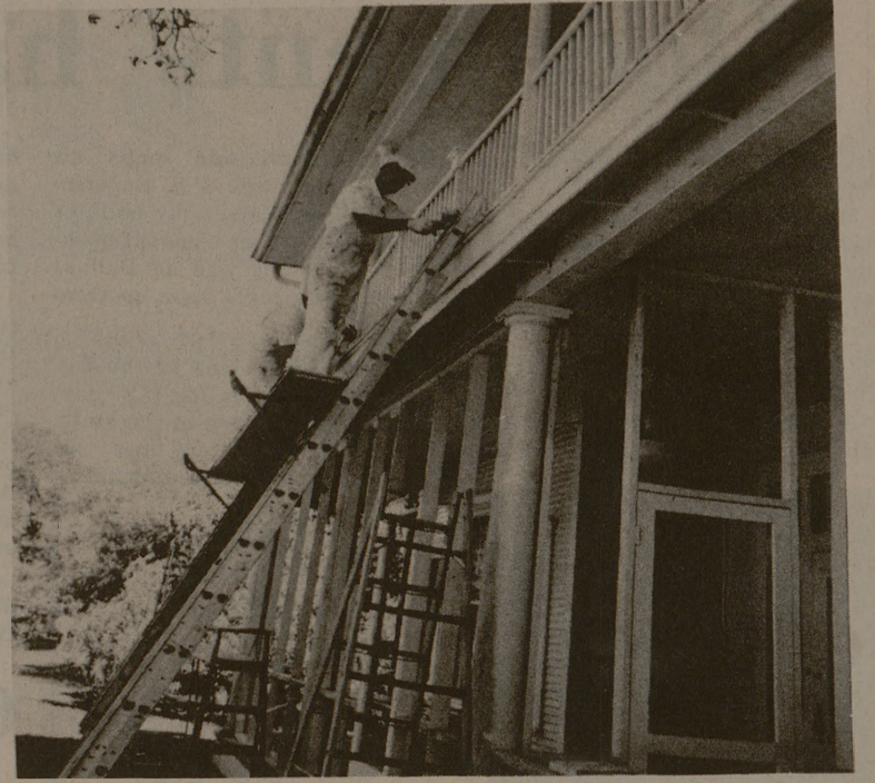
PHYSICAL PLANT craftsmen prepare the old TAMU Board of Directors building for use as headquarters of the new Texas A&M University Press.
