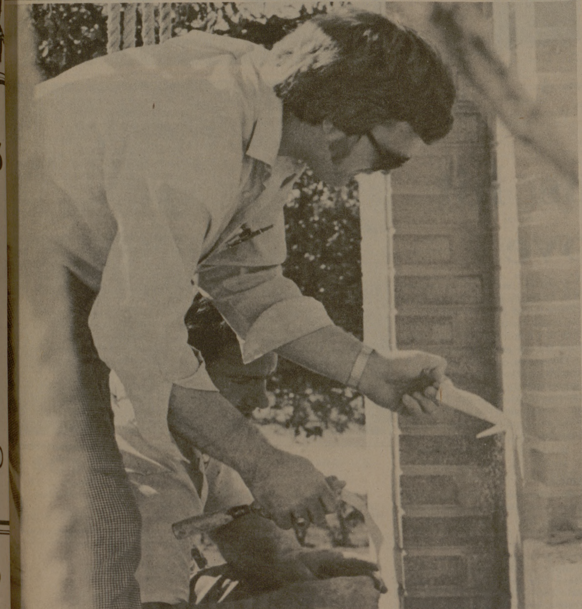
NOTHING UNDERNEATH the masking tape John Hollaway is pulling off Sbis Hall. He and fellow-worker Peter Adams are merely patching leaks, from a 12-foot high scaffold, in the old building. The masking tape is applied to bricks prior to caulking. (Photo by Gary Baldasari)
