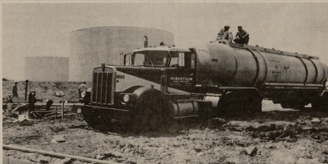
TRUCKERS HAVE BEEN busy lately filling TAMU's two new one-million-gallon fuel oil storage tanks on Finfeather Road. The tanks represent almost a month's supply of fuel for campus power system and will be used to hedge against another episode of the energy crisis. (See story page 5)
