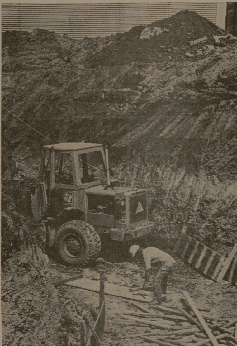
CONSTRUCTION CONTINUES for the burial of two small fuel tanks near the University Laundry. Two million-gallon tanks have also been buried near Finfeather Rd. in anticipation of a winter energy crisis.
