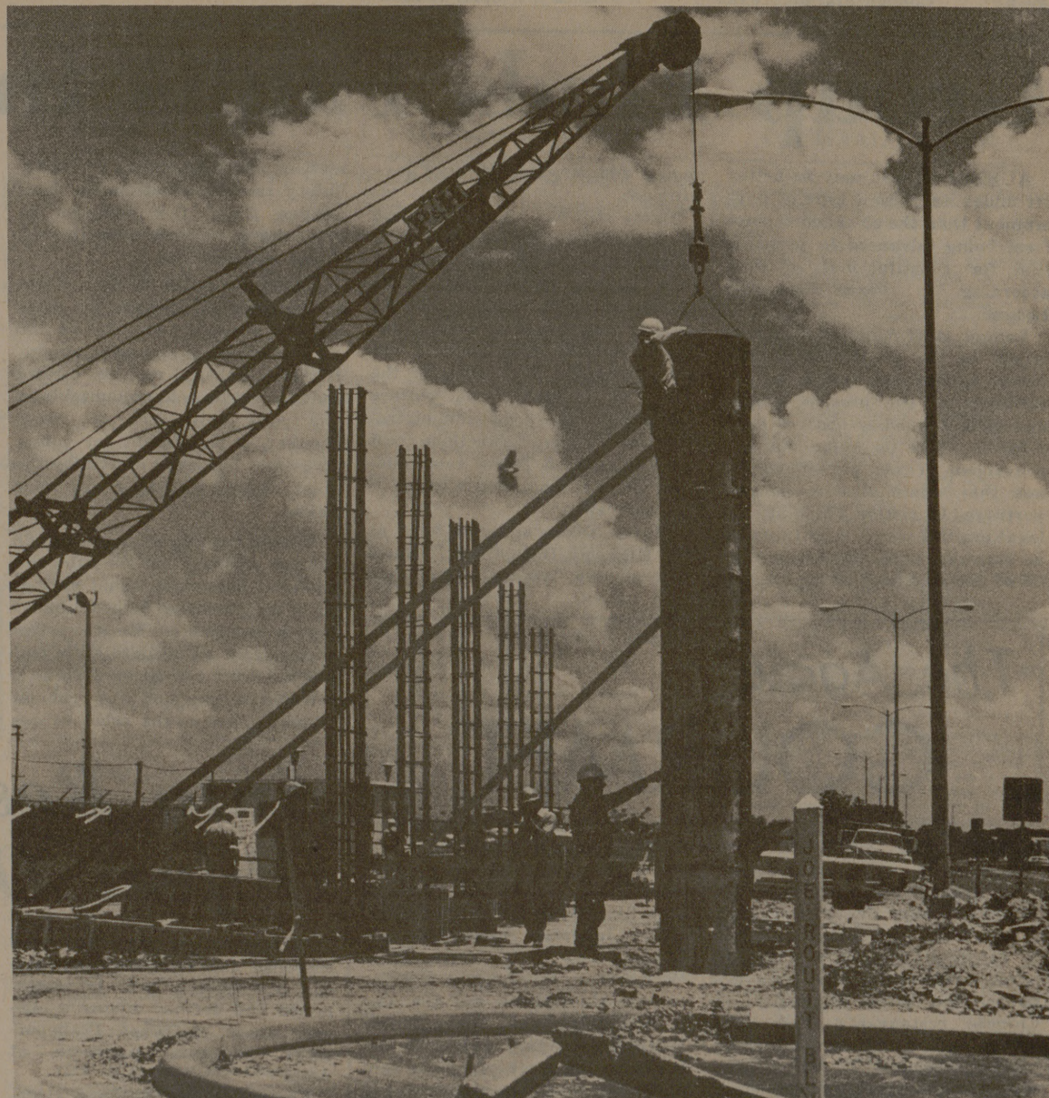
CONSTRUCTION BEGINS on overpass-walkway by the pool. The structure is scheduled for completion this fall.
