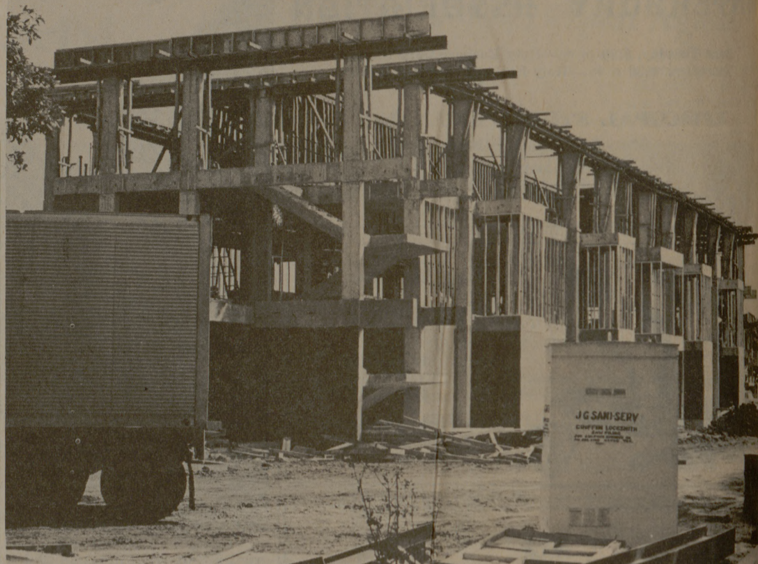
THE HOME FOR UNWED JOCKS—The new $3.4 million athletic dormitory is finally taking shape with a scheduled completion date of Jan. 1. All single full scholarship athletes will be housed in the two-wing three-story structure. A single one-story commons area will separate the two wings. It will have a 200-bed capacity. (Photo by Peter Leabo)
